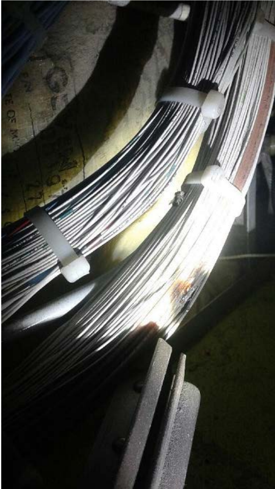
Arcing evidence on wires
