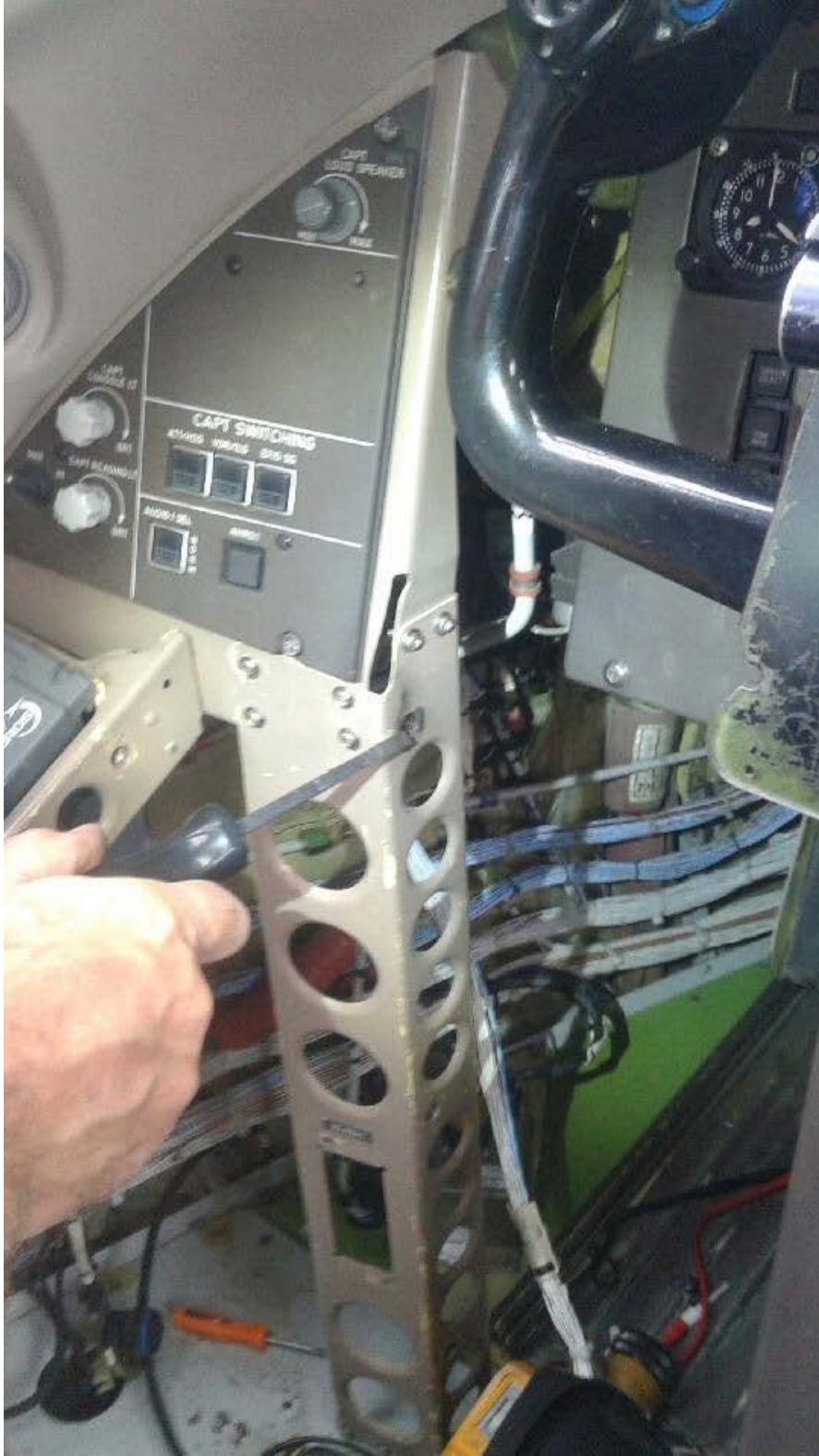
Location of fastener and evidence of arcing
